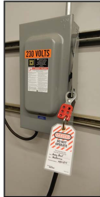
Figure 1: Lockout/Tagout on the Power Source Panel
